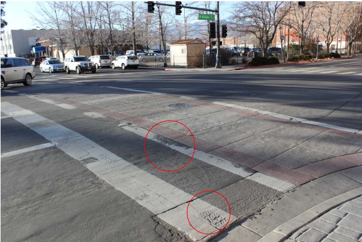
Photo 30 – Showing an example of pavement markings that should be replaced.
