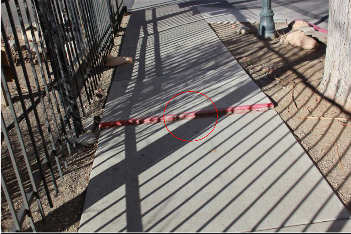
Photo 34 – Showing an example of a section of sidewalk that has heaved.
