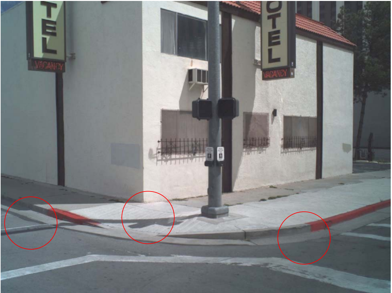
Photo 32 – Showing the lack of tactile strips on a pedestrian ramp and the ramp not aligned to the crosswalk to the right at the intersection of Arlington Avenue and 5 th Street.
