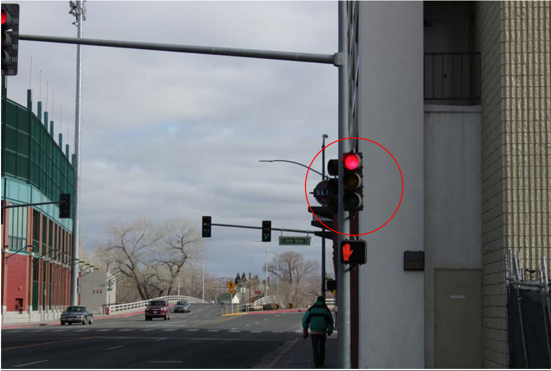
Photo 14 – eastbound at the intersection of 2 nd Street and Evan Avenue showing that there is a back plate missing on the signal head.
