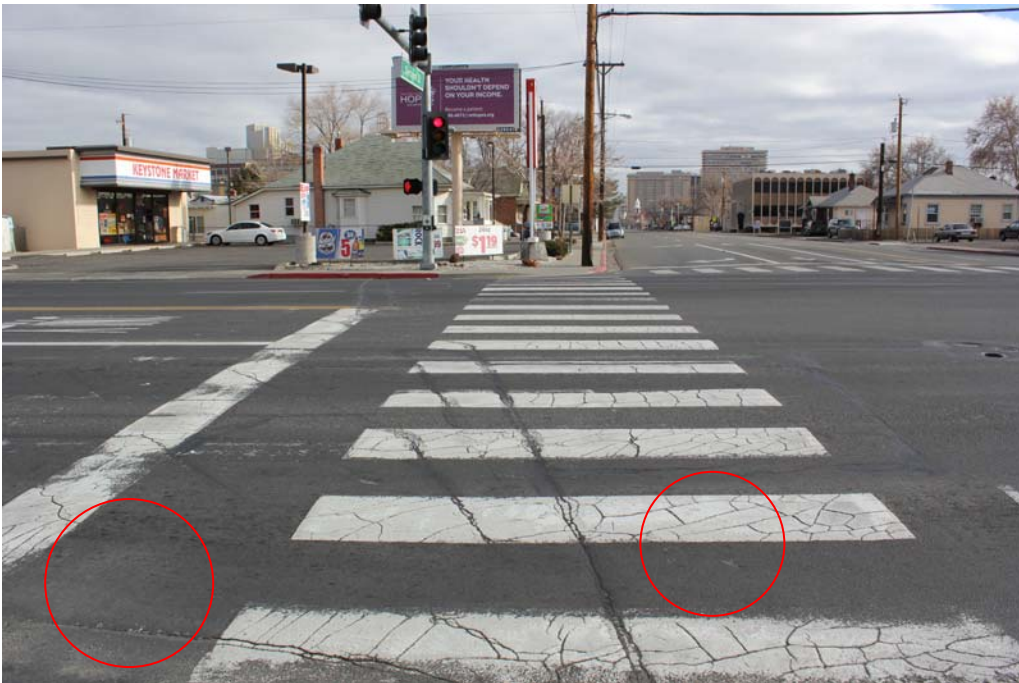
Photo 2 – Showing an example of pavement markings that should be replaced.
