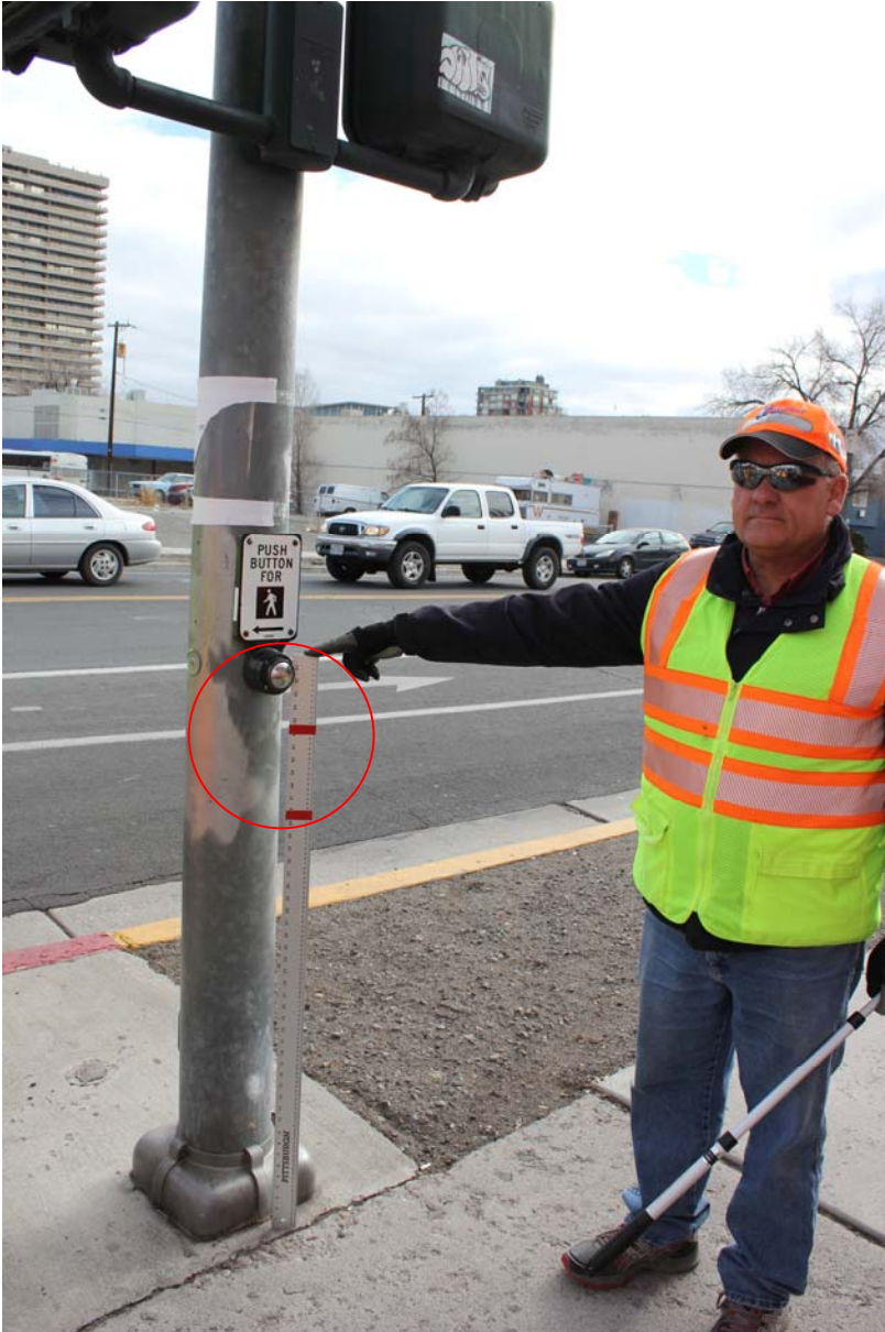
Photo 31 – Pedestrian Push Button is located above the 42 inches maximum height above the sidewalk.
